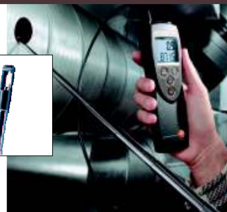
Monitoring air velocity in air conditioning ducts
